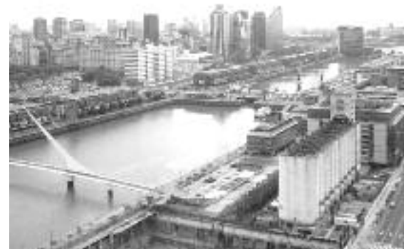
Figure 19. Puerto Maderos under construction, view towards Santa Catalinas. The highway La Plata- Buenos Aires along the river-side isolates Puerto Maderos. Source: A. Arrese, 2007
